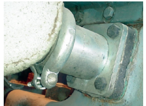
Old, rigid water inlet header
