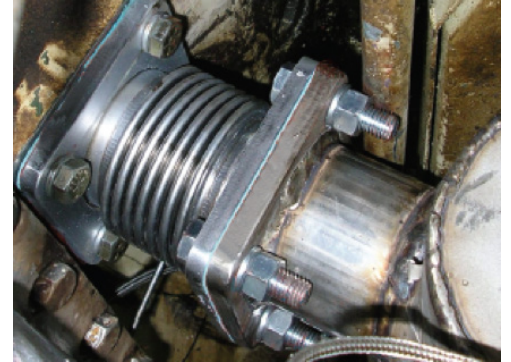
New, flexible water inlet header
