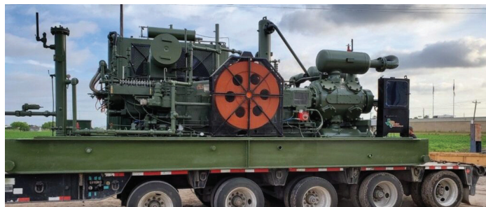
Leased AJAX® DPC-2802 LE Integral Compressor Package
