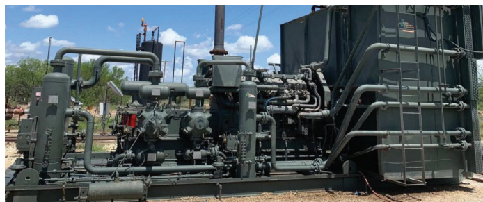
Leased CAT 398TA Compressor Package with Ariel Frame
